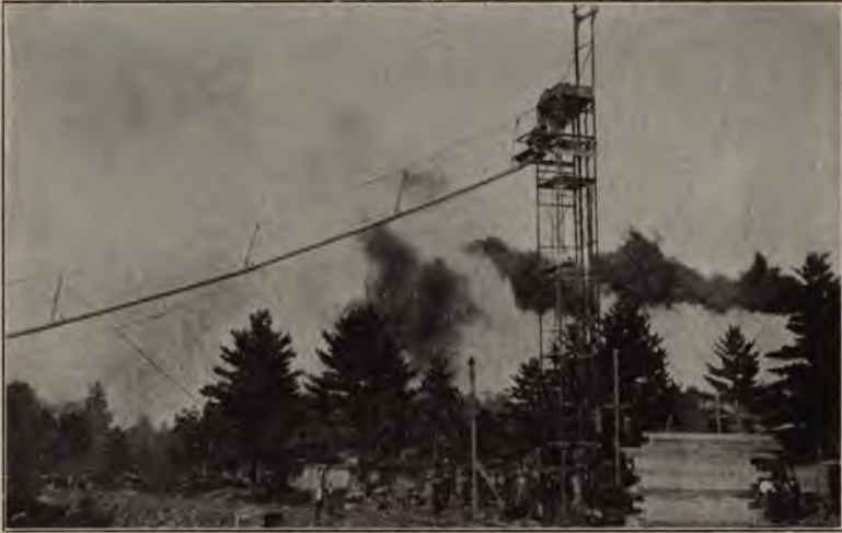
Peninsular Power and Development Co. Constructing Dam at Twin Falls near Iron Mountain, Mich.
